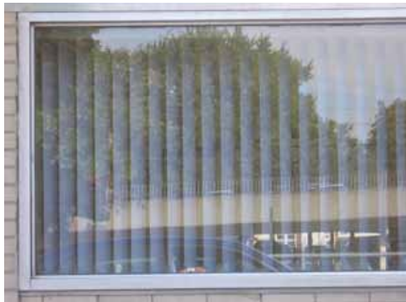
While patterns on the exterior surface of glass are most effective, blinds and curtains can help disrupt reflections. Partially open blinds, like those seen here, are most effective. Photo: Christine Sheppard, ABC
