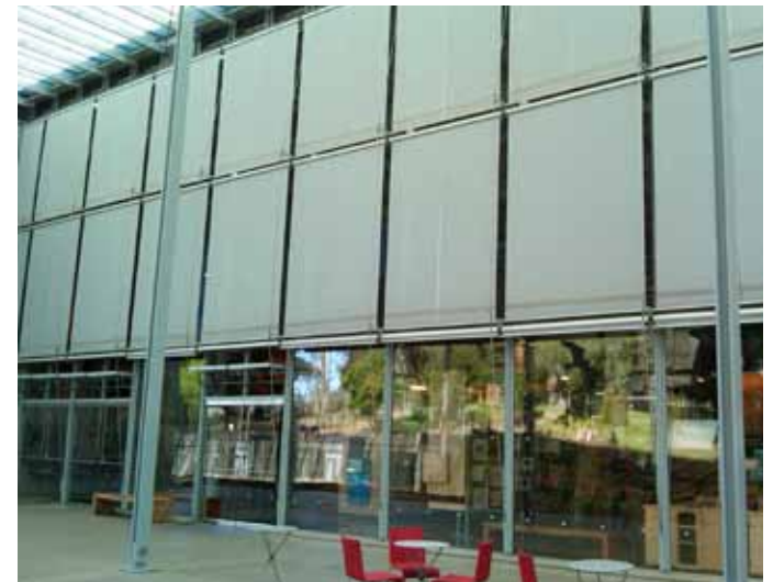
External shades on Renzo Piano's California Academy of Sciences in San Francisco are lowered during migration seasons to eliminate collisions. Photo: Mo Flannery
