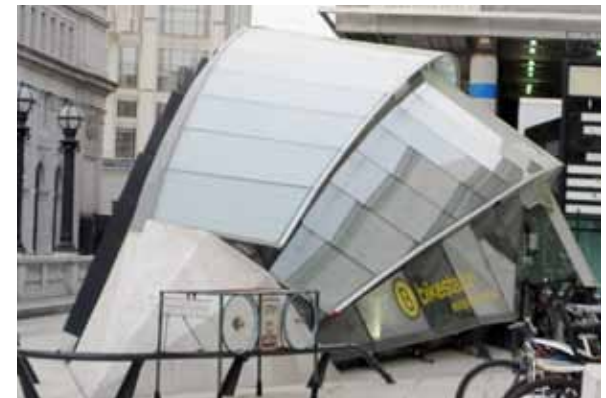
A dense internal frit pattern on the glass of the Bike and Roll building, near Union Station in Washington D.C., makes it look almost opaque. Photo: Christine Sheppard, ABC
